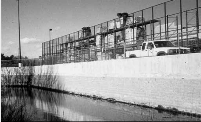
When there is no room to set guide rails behind a wall, traffic barriers can be placed directly on top of a wall.
