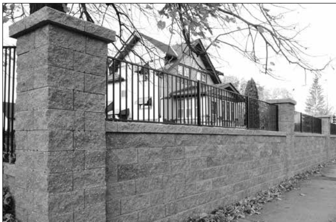
Railings between columns provide attractive fall protection.
